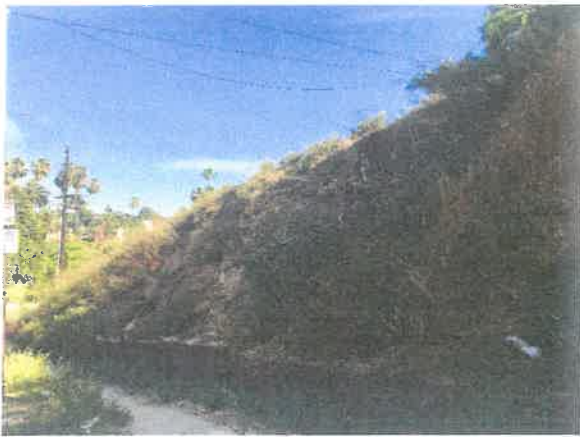
Figure 5: Northerly Property Line Depicting Slope Greater than 60% and Failing Hillside
