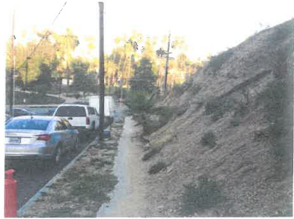
Figure 6: Northerly Property Line Depicting Slope Instability and Erosion
